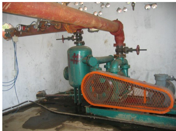
Figure 1: Drainage pump of Coal Mine A
